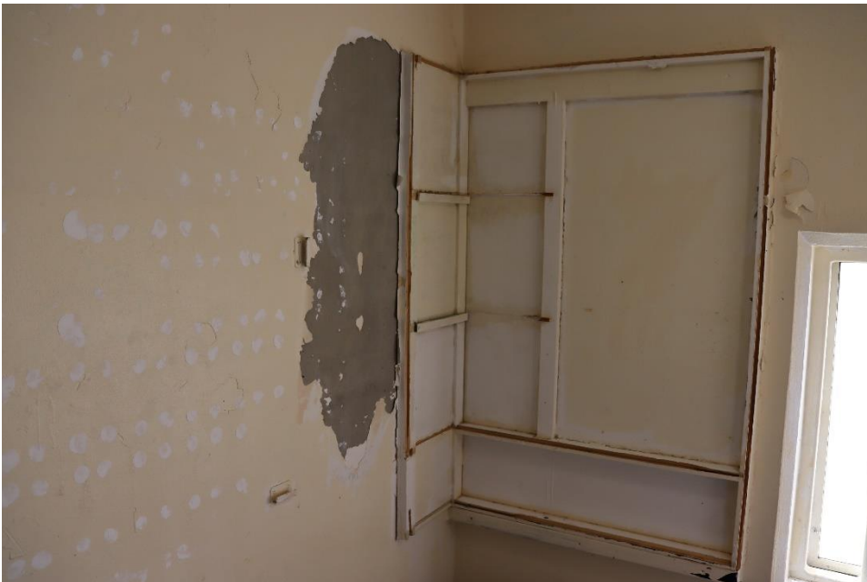
A cell with a wall unit missing
