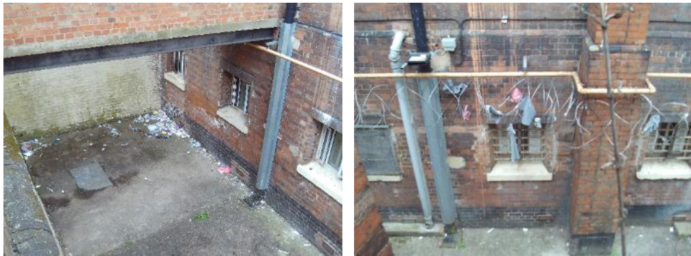
Litter in outside gulleys and wiring
