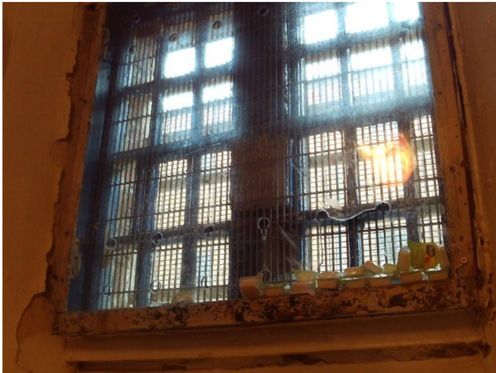
Cell window with damaged plastic cover
