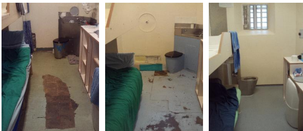
Cells in worn condition (left and middle) and refurbished cell on the Parsons unit (right)
