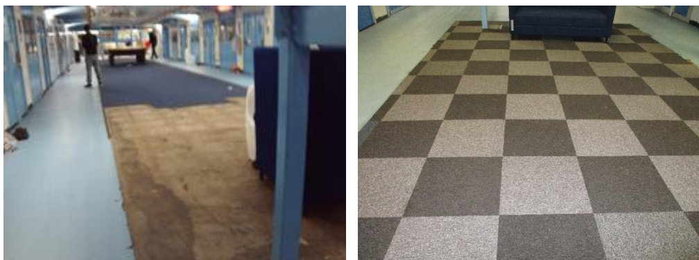
Damaged flooring on houseblock one south at the time of the inspection in February 2025 (left) and repaired flooring on houseblock one south at the time of this visit.
